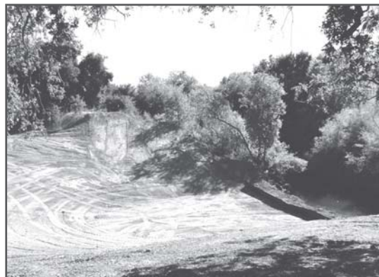
These cut slopes along the river have now had erosion control fabric added and are being revegetated next month.
