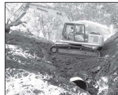
Heath Garman compacting soil over a newly placed culvert. The old culvert was replaced because it was too narrow and wasn't in line with the natural stream channel.
